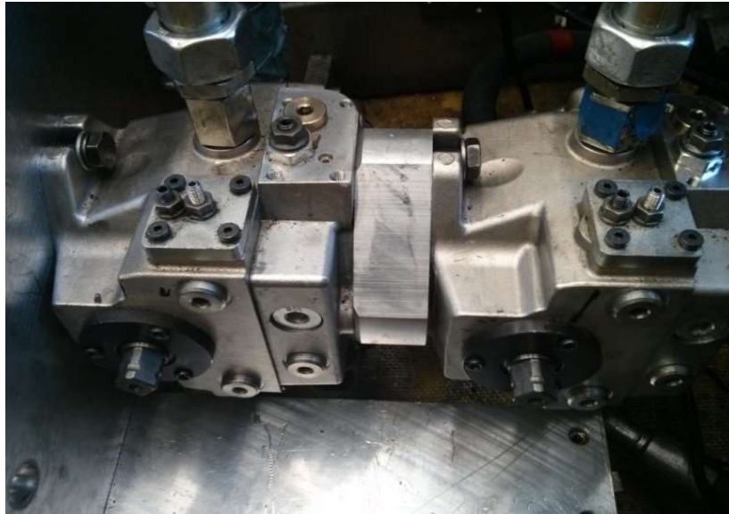
Figure 3.7 The Hydraulic Pumps
