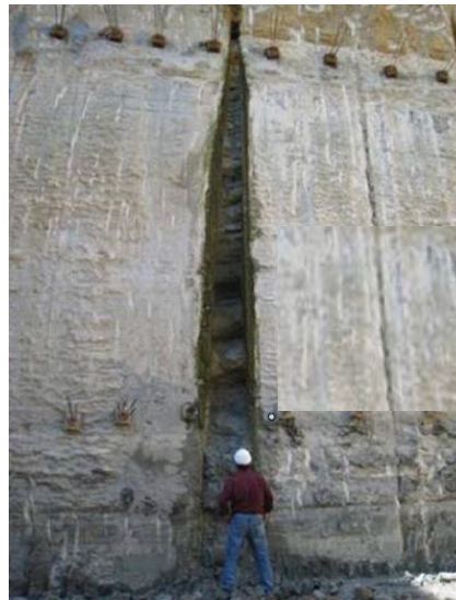
Figure 1.4: Wall damage due to column deviation during the deep soil mixing process. Courtesy: Deep Foundations Institute, TreviGroup [3].
